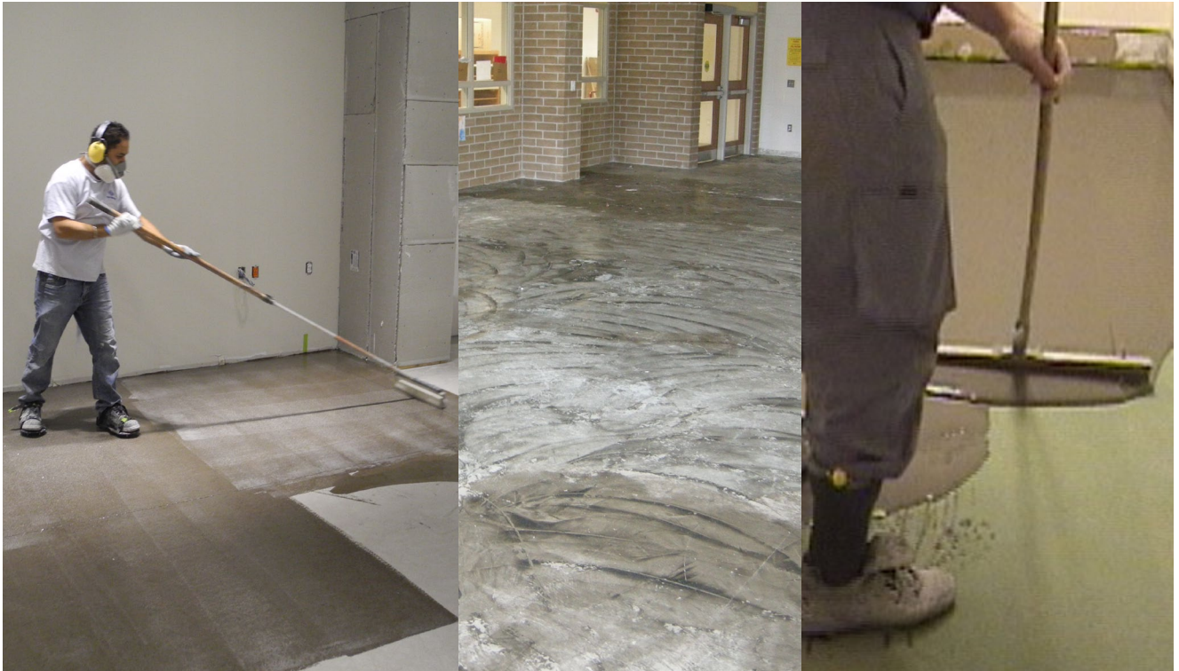
Left: Epoxy application for moisture control on new concrete floor. Centre: Moisture damaged floor at high school. Right: Concrete overlay going over epoxy moisture control coated floor.
