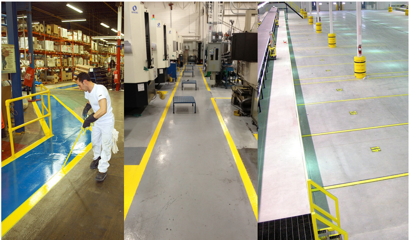
Left: Blue walkway with applied yellow safety lines in Sonoco manufacturing facility. Centre: Epoxy safety lines designating walkway areas in Exco facility. Right: FedEx warehouse yellow epoxy walkway safety and truck parking lines.
