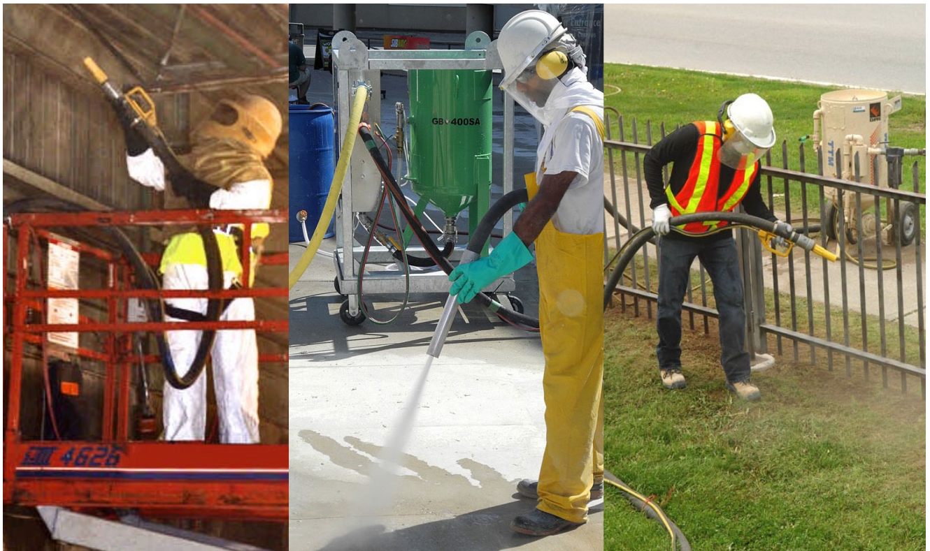
Left: Rusted and peeling metal ceiling deck in factory being sandblasted. Centre: Abrasive blasting to remove gum and dirt from concrete walkway. Right: Rusted metal fence surface being sandblasted to prep for painting.
