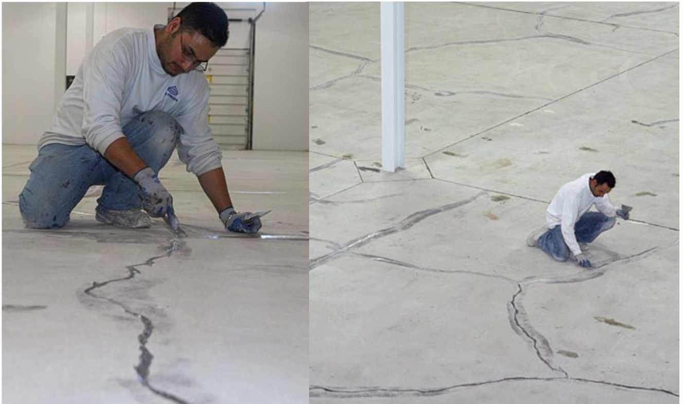
Cracks being filled and patched after completion of crack chasing work to prep cracks on older concrete floor.
