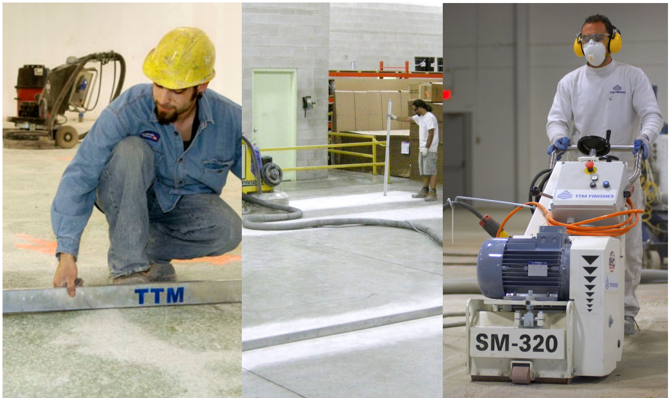
Left: Grinding concrete to level floor for tile installation. Centre: Using laser measurement to achieve superflat floor tolerances for automated racking system installation. Right: Concrete Shaver milling a concrete floor.
